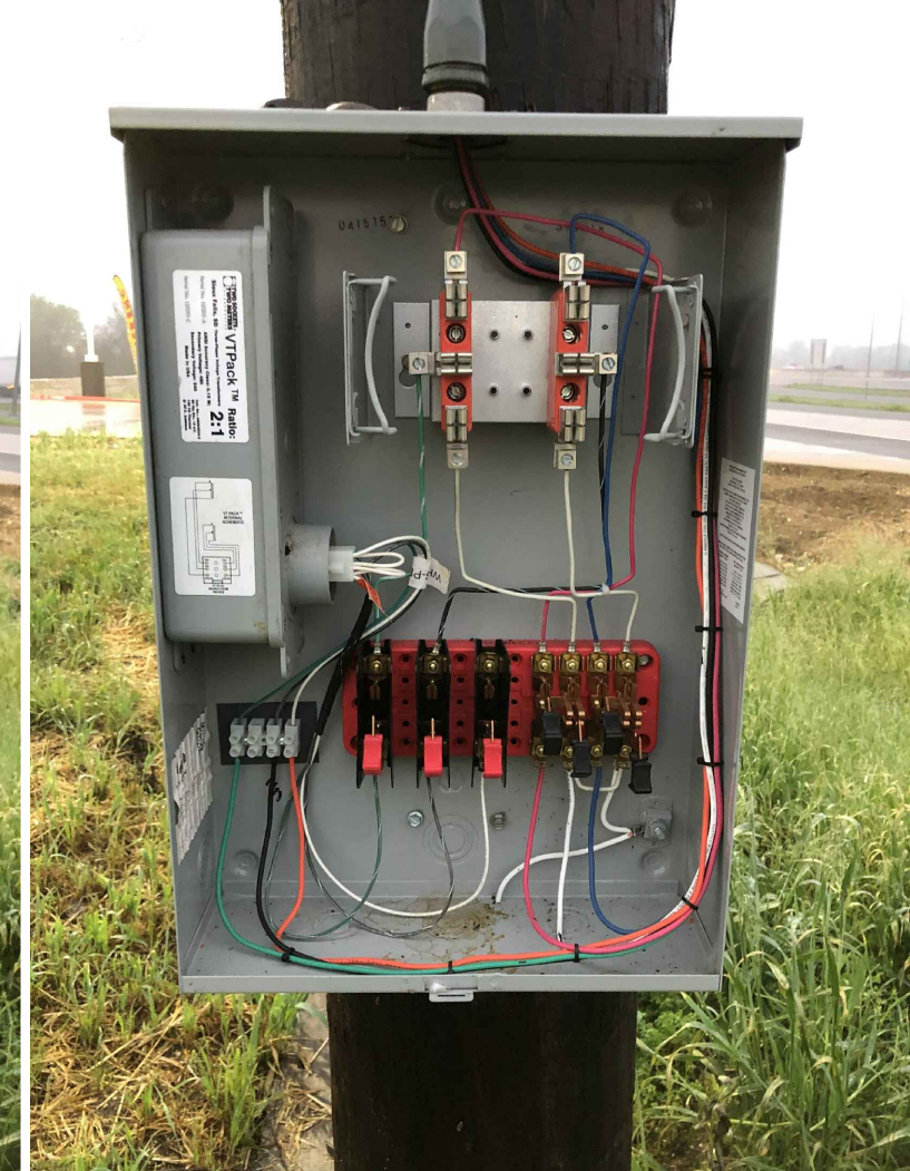
METER NOT INSTALLED
